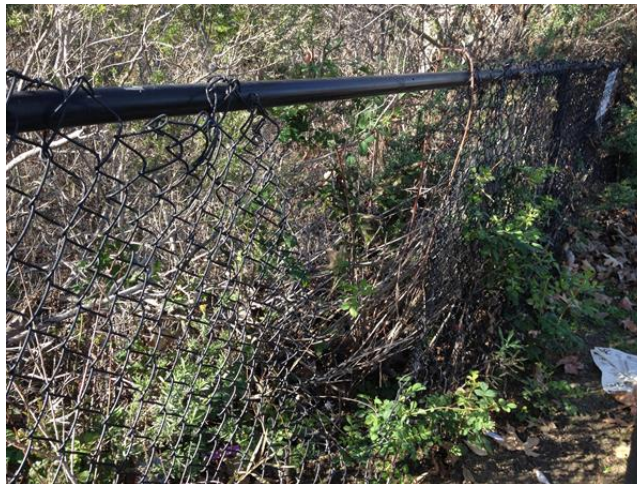
Photo 9: Tear in fence at corner of El Camino Real and Town Center drive
