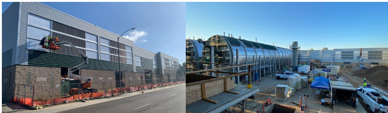
Photos from May 2020 and June 2020 of EDCO's Anaerobic Digester Facility
