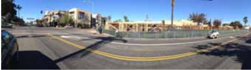
A panoramic shot on Adams Avenue shows Kensington Commons under construction between Marlborough Avenue and Edgeware Drive. Roger Showley
