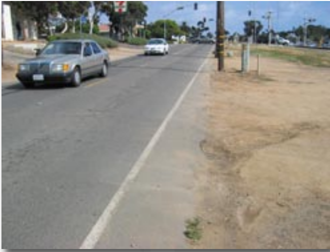
Vulcan Avenue - Uneven pavement edge with minimal shoulder
