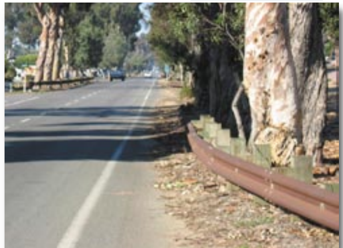
Coast Highway 101 - Guardrails and eucalyptus in close proximity to the traveled way
