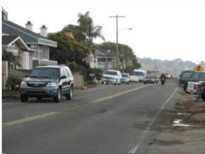
San Elijo Avenue - Crumbling pavement edges correspond with off-street and on-street parking
