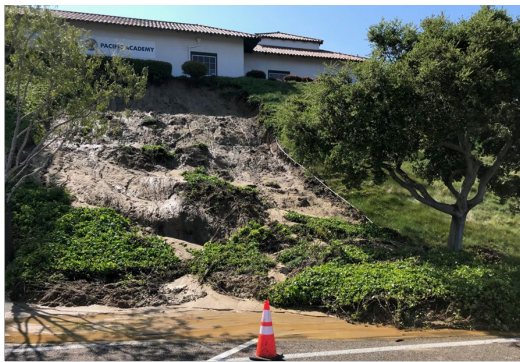
Surficial Slope Failure Caused by Heavy Rain
