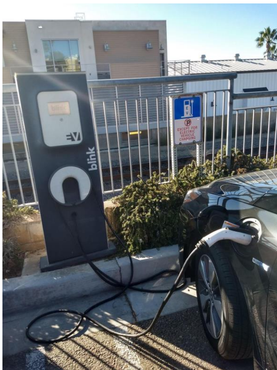
FIGURE 11: EXISTING LEVEL 2 EVSE IN ENCINITAS
