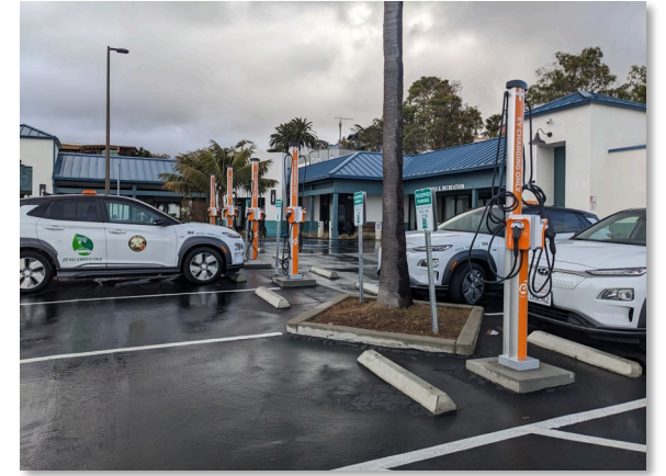
EV Charging Stations, 2022
