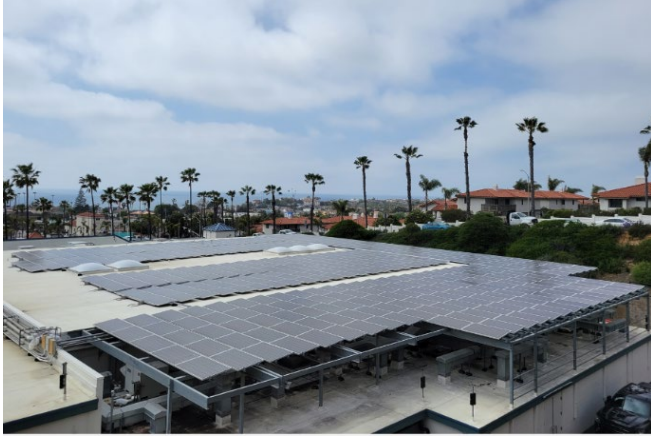
Solar Panels on City Hall Roof, 2008
