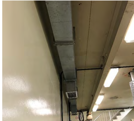
Figure 2.13: Existing Air Supply Ducting and Vents on 1 st Floor
