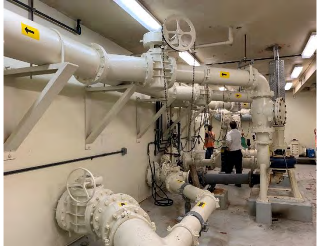
Figure 2.7: Existing Pump Discharge Piping Assembly
