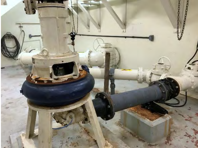
Figure 2.6: Existing Pump #3 Modified Suction Assembly
