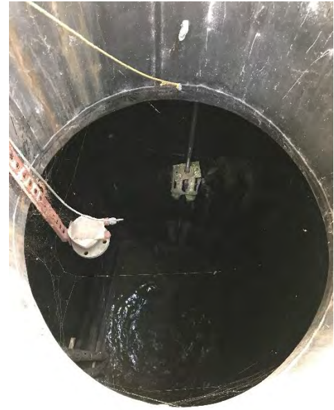
Figure 2.10: Moderate Corrosion on Existing Ultrasonic Level Sensor Mount
