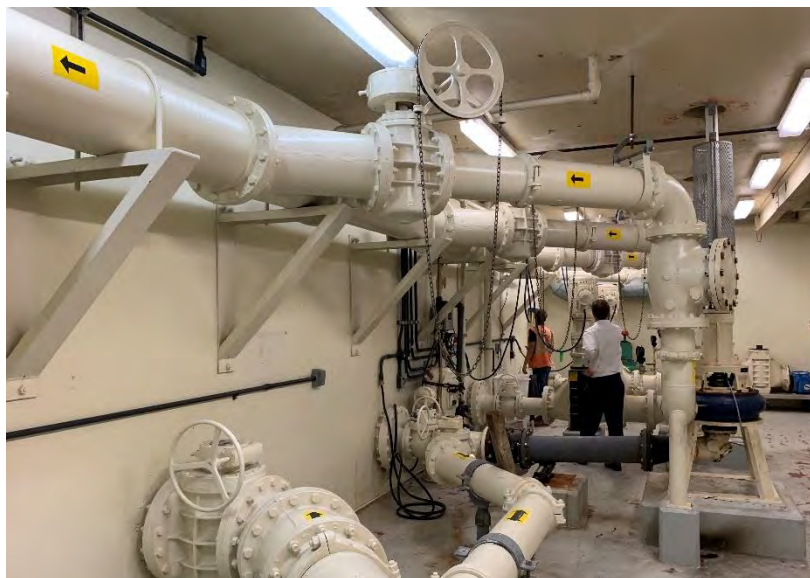
Figure 2.1: 1 st Floor Existing Pumps and Discharge Piping Manifold
