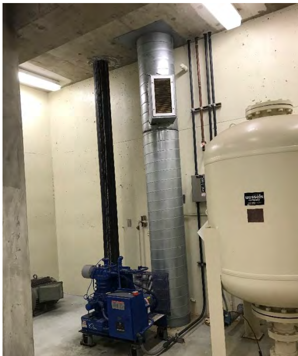
Figure 2.16: Existing Air Exhaust Ducting and Vent on West Wall of 2 nd Floor
