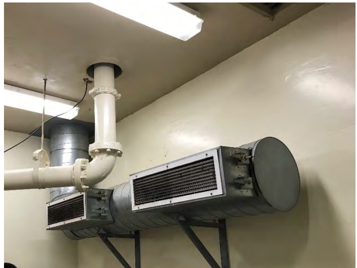
Figure 2.17: Existing Air Exhaust Ducting and Vents on West Wall of 1 st Floor
