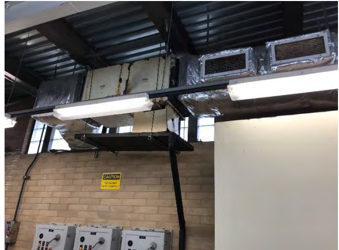
Figure 2.11: Existing Inline Air Supply Fan, Filter Box, and Ducting on North Wall of 3 rd Floor
