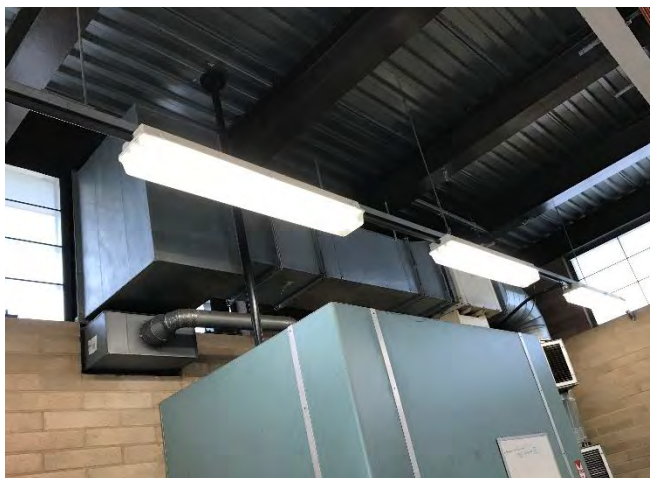
Figure 2.14: Existing Air Exhaust Fan and Ducting on South Wall of 3 rd Floor
