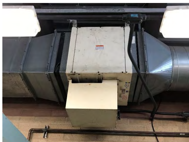
Figure 2.15: Existing Inline Centrifugal Air Exhaust Fan South Wall of 3 rd Floor
