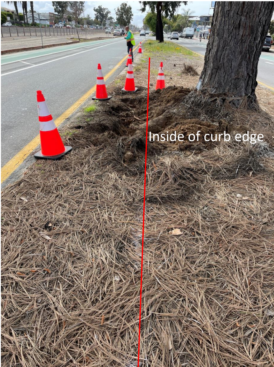
25753ETree : Detail view of root excavation down to 6 inches below finished grade
