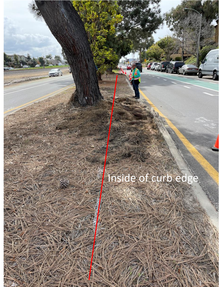
25725Etree : Detail view of root excavation down to approx. 6 inches below finished grade
