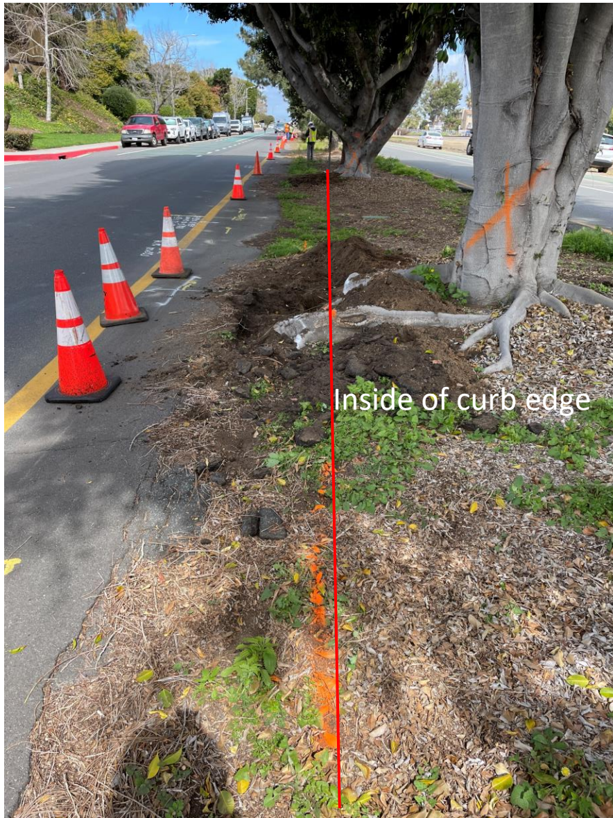
25735E Tree: Detail view of root excavation down to approx. 6 inches below finished grade
