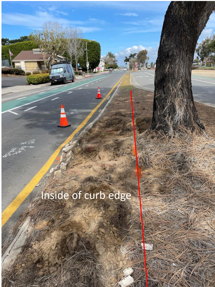
25725E Tree: Detail view of root excavation down to approx. 6 inches below finished grade
