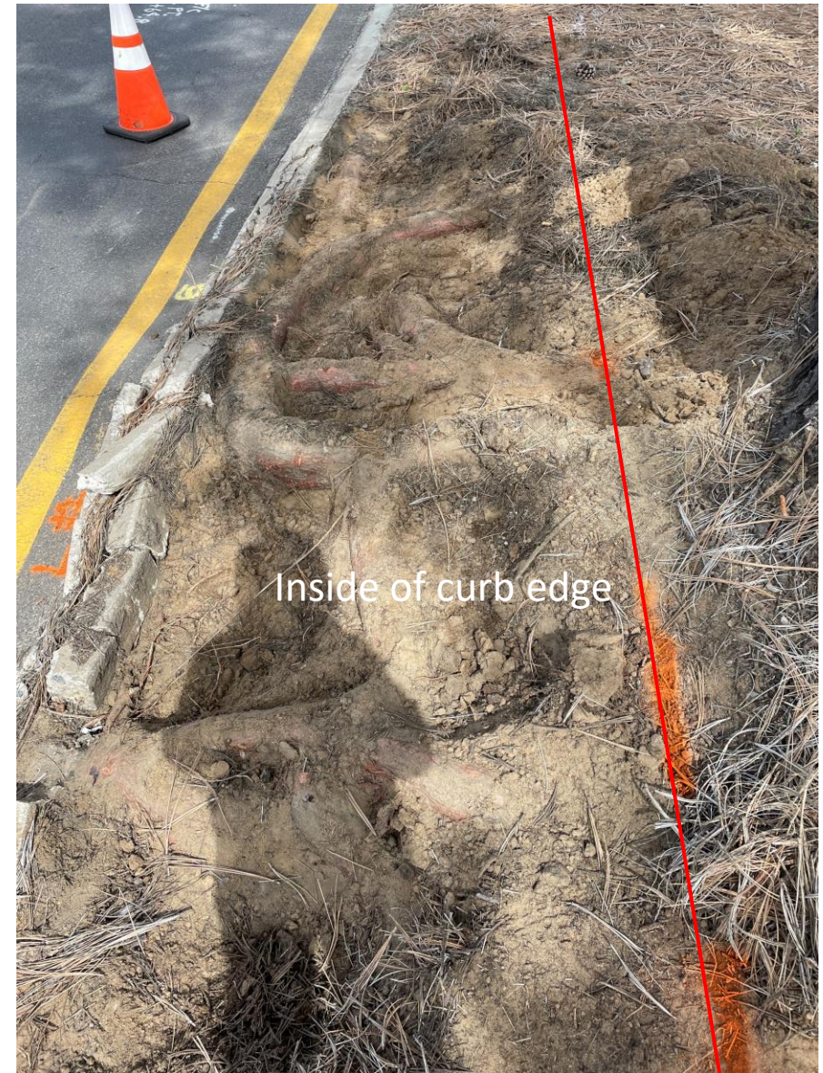
25725E Tree: Detail view of root excavation down to approx. 6 inches below finished grade
