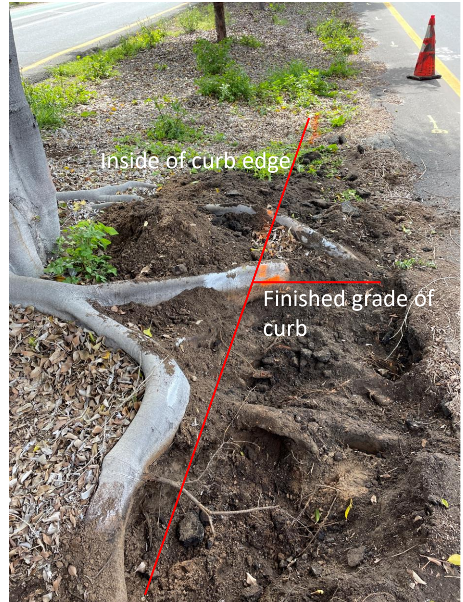
25735E Tree: Detail view of root excavation down to approx. 6 inches below finished grade
