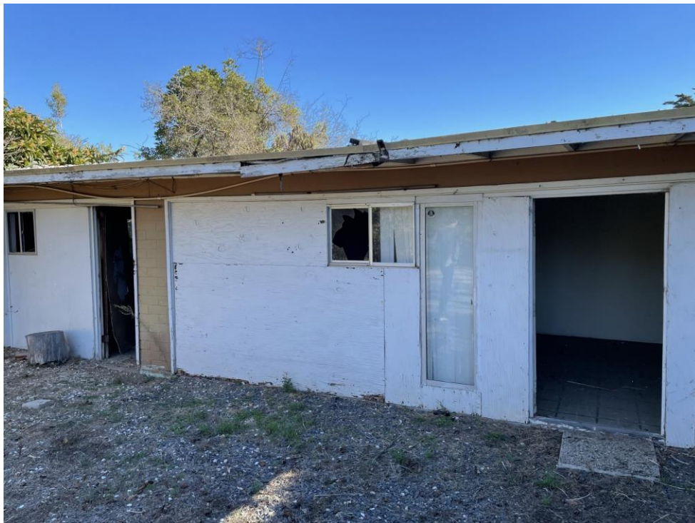
Photograph #12 Dilapidated residence at 1190 Island View Lane.
