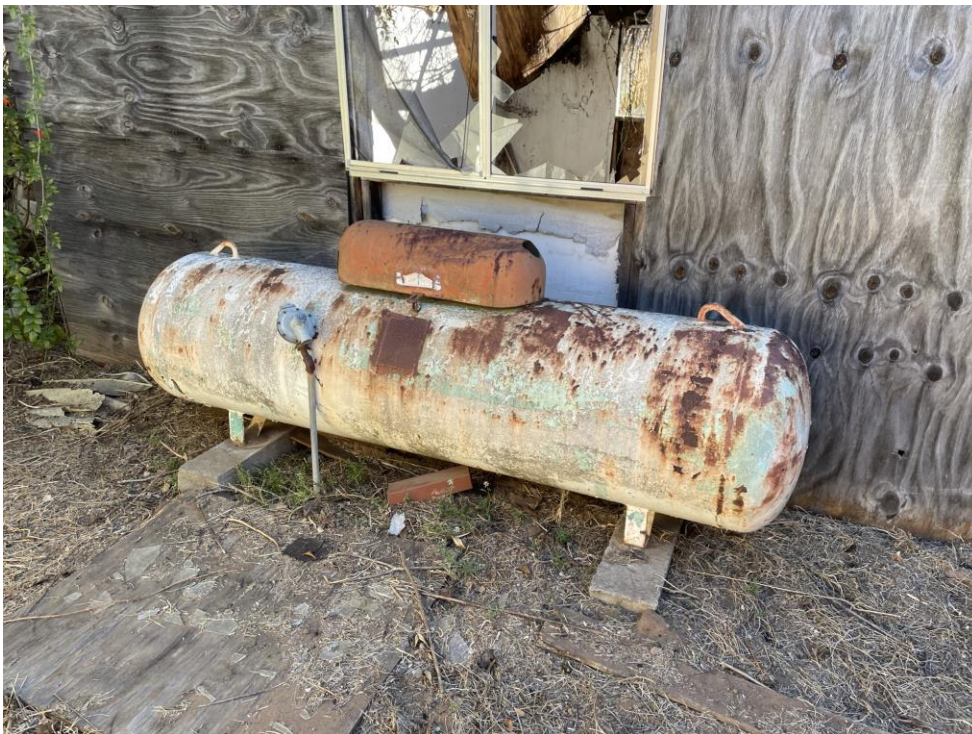
Photograph #14 Propane tank on exterior of residence at 1190 Island View Lane.
