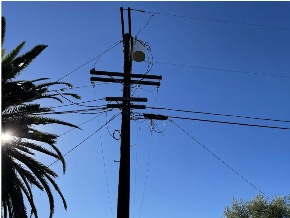
Photograph #16 Pole-mounted transformer in northern portion of the Site.
